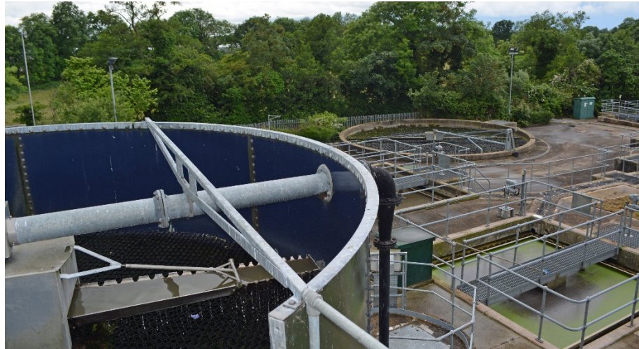
Two stage trickling filter process at Ballinderry WWTW
