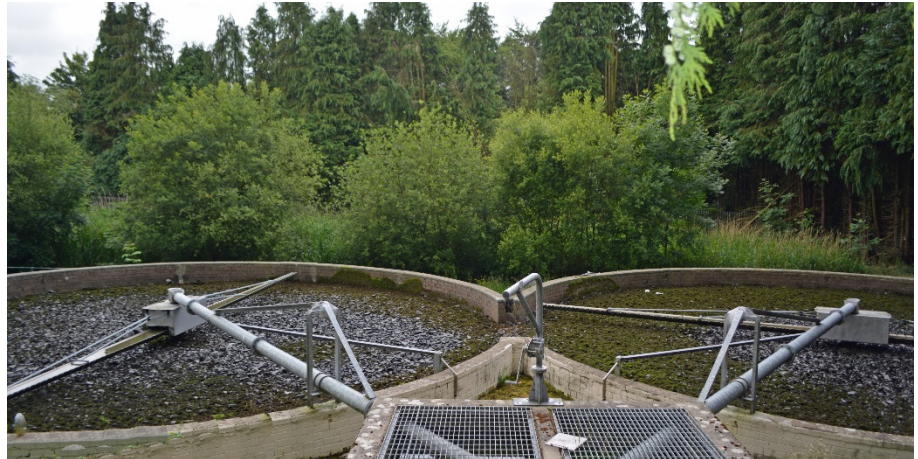
McGill Distributor and Reed Bed at Lawrencetown WWTW
