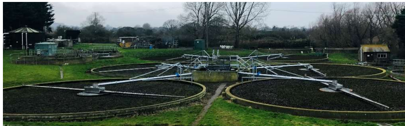
McGill Distributor installation at Neaves Lane WwTW
