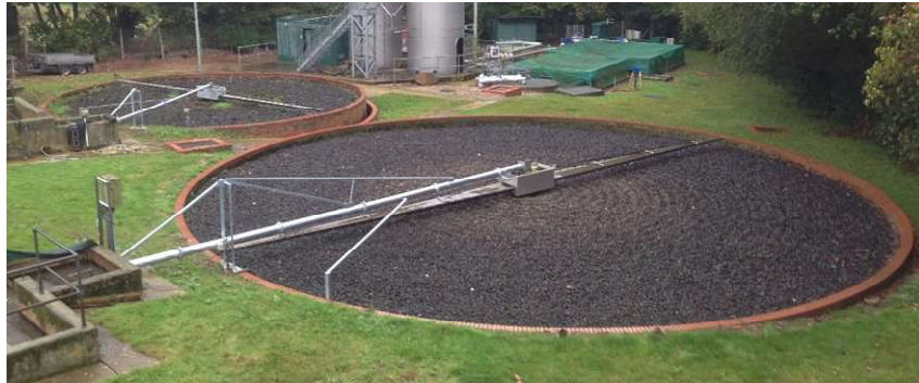
McGill Distributor installation at Guestling Green WwTW
